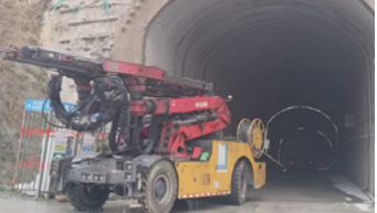
Zhejiang Tiantai Pumped Storage Power Station
